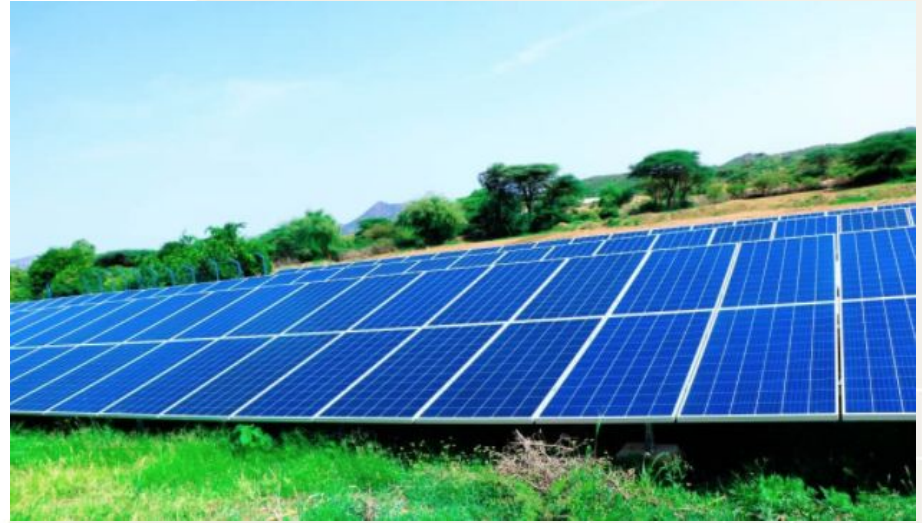
Solar installation at SHABA Water. Photo by Said Abib, KAAFI Solar
